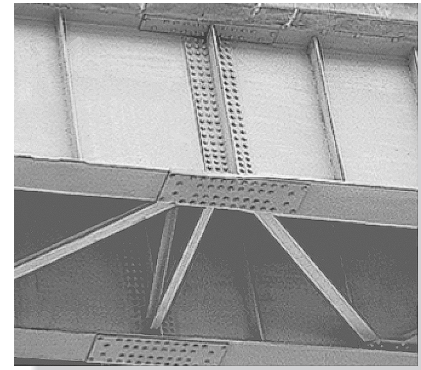
Shown are typical splice plate joints used to connect the steel girders of a highway bridge.
